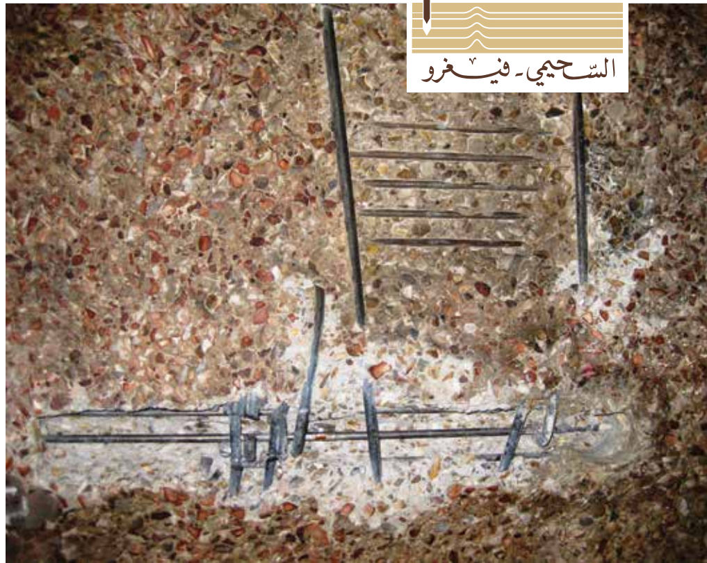
Spalled surface affected by heating exposing pre-stressed tendons.
